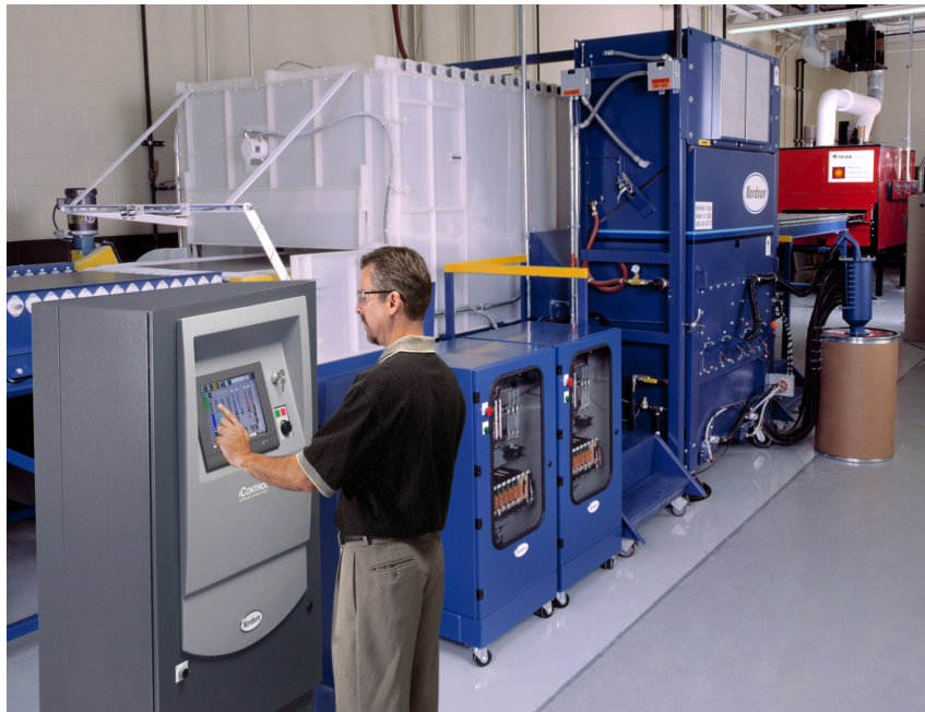
Nordson® flat-line powder coating system.
